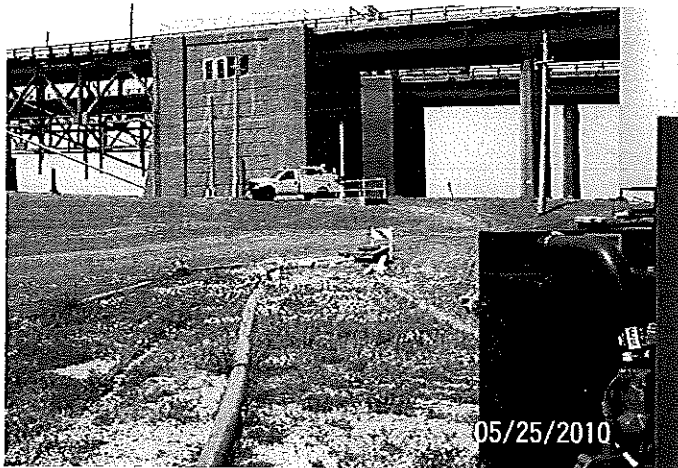
Three pumps east of Interstate 74 bridge near the levee
