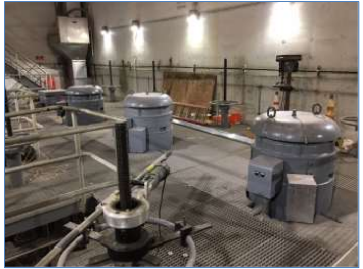
Raw sewage pump motors
